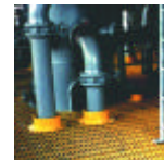
FIBERGLASS PIPE PENETRATION COLLARS
